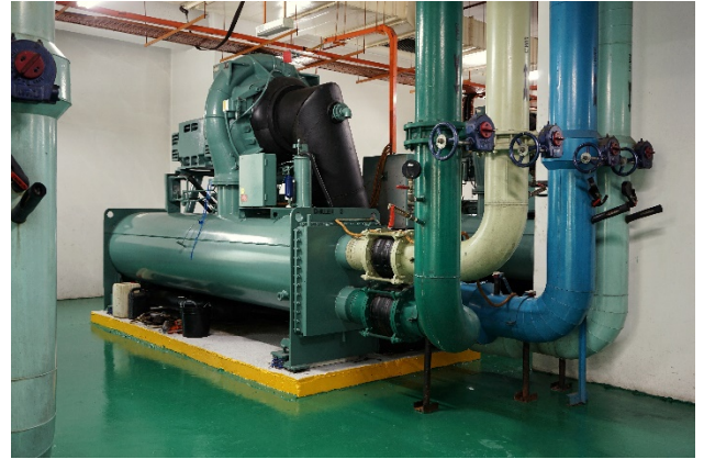
HCFC-123 centrifugal chiller.
