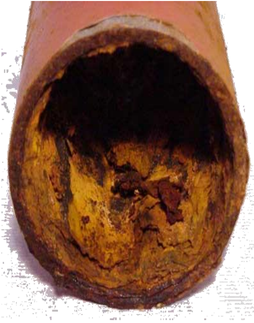
Rusted iron water pipe
