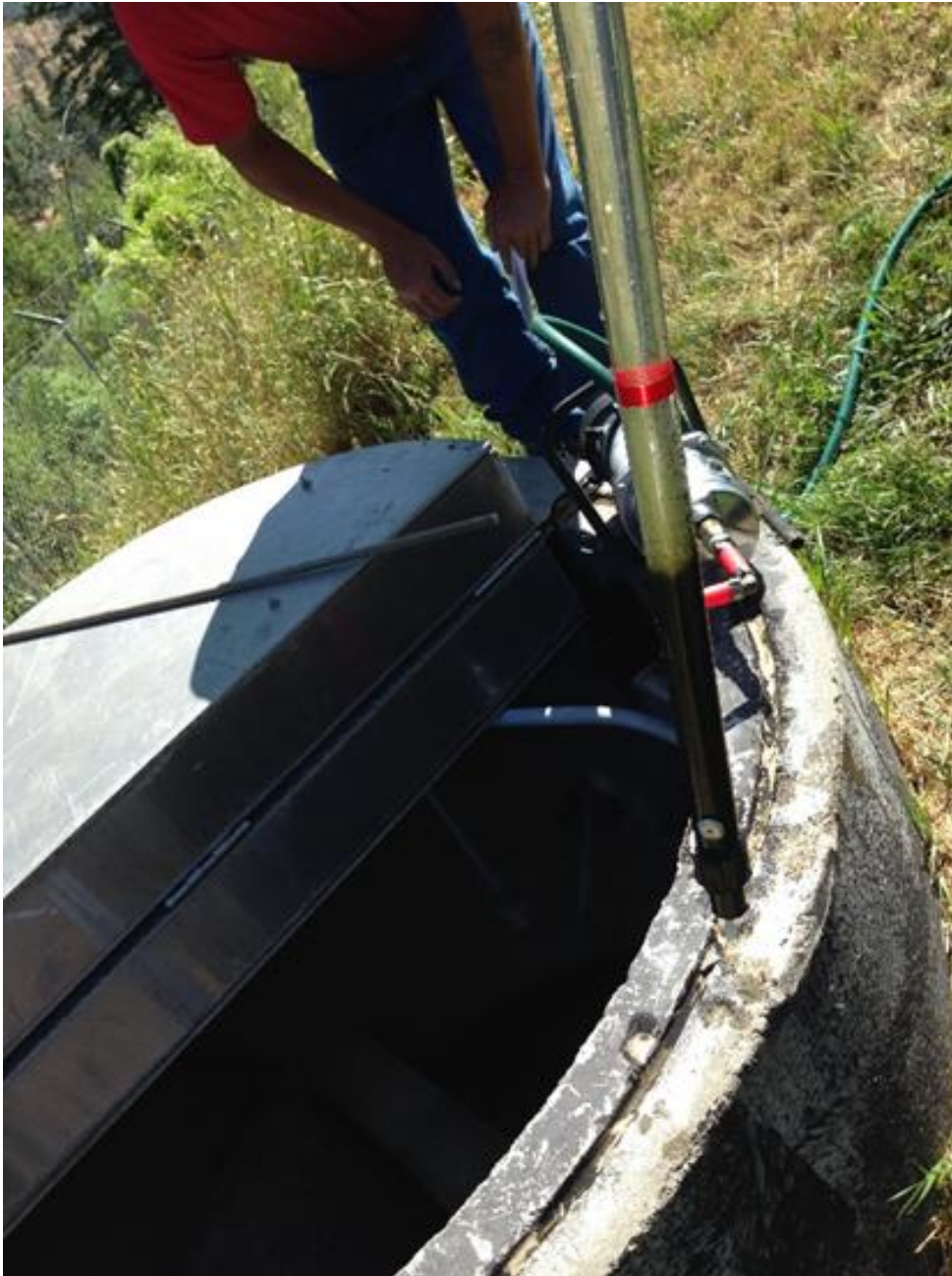
Sludge in the Discharge Well
