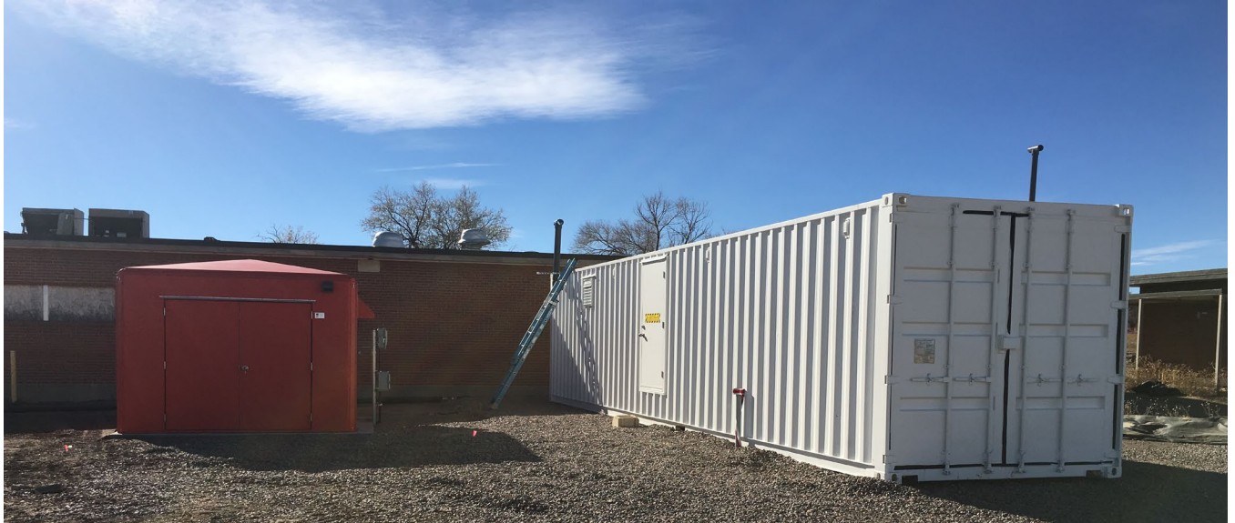
Figure 3 – Downing Reservoir Groundwater Treatment Plant
