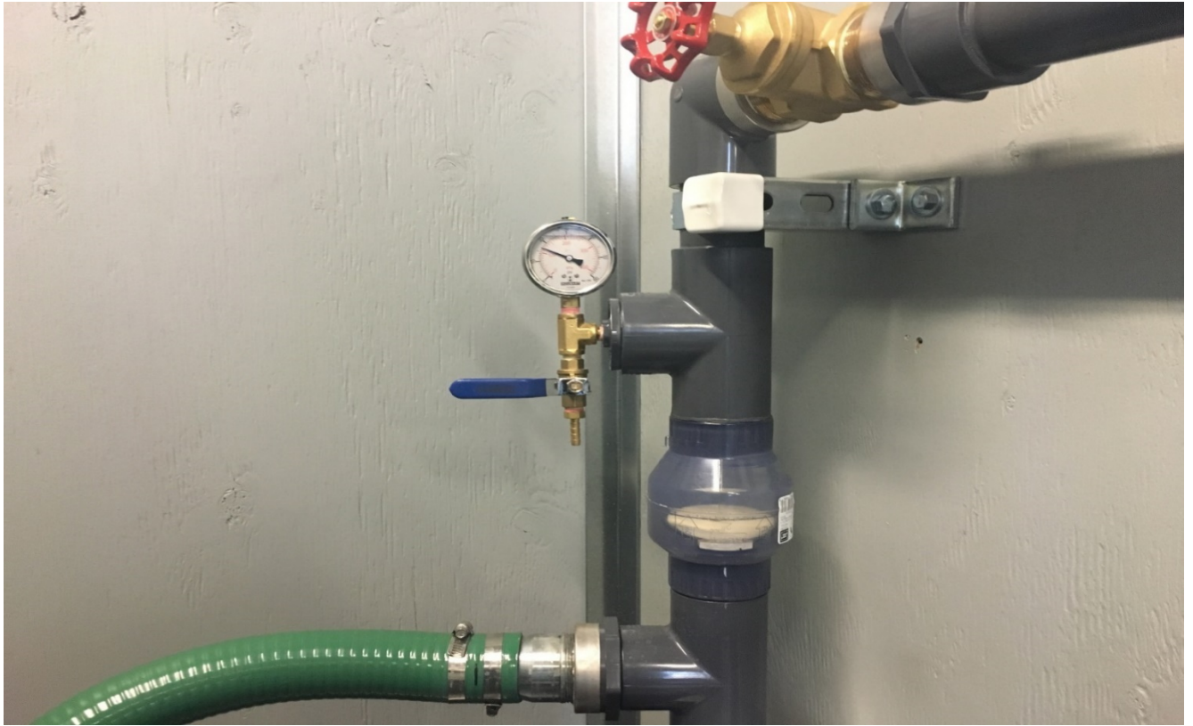
Figure 4 – Outfall 001B/Effluent Sampling Port
