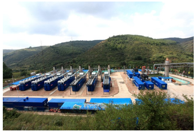
Exhibit 4. Duerping Mine Flare, Shanxi Province, China (Courtesy of Sindicatum Sustainable Resources)
