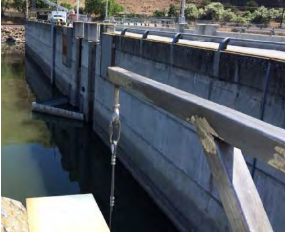
Figure 3-3. North of the John Day South Fish Ladder Exit: Steel Bracket Mounted to Dam Structure to Allow Temperature String to Hang Freely at Bottom of Structure.
