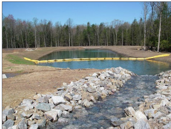
Figure 3. The Oneida #3 treatment system discharges through a limestone channel into a settling pond.
