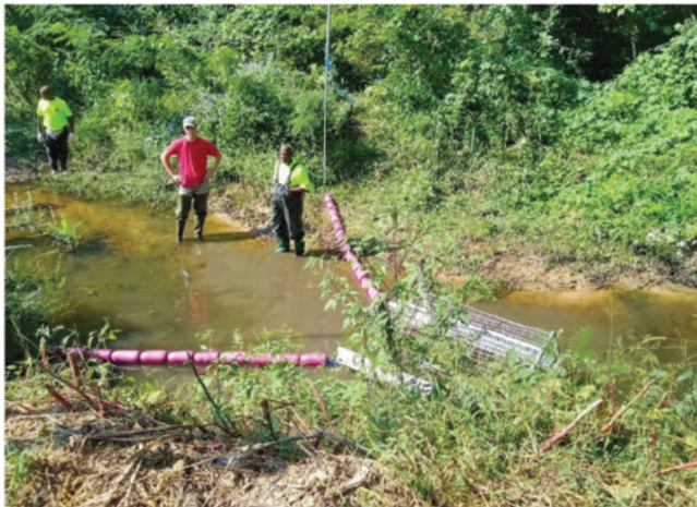
Installation of a Litter Gitter, or trash trap, installed along a creek in the U.S.
