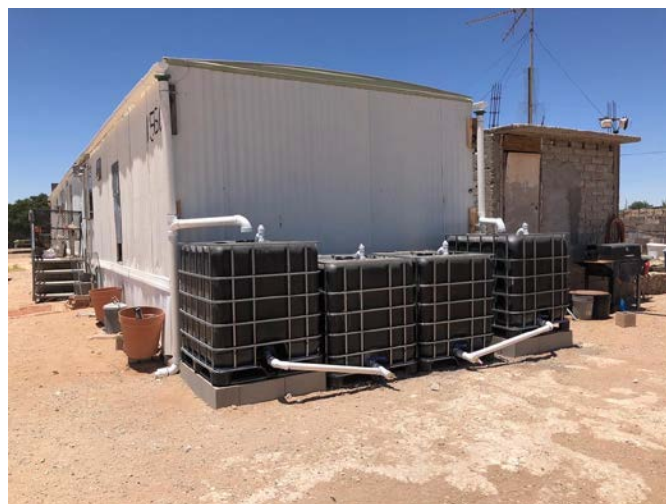
Figure 1. Rainwater harvest system at mobile home in Cochran Colonia, El Paso County, Texas.
