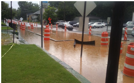
Boone Green Street under construction. A recent rain highlights the need for this project. The green street project combined with Rodney Cook Park and Boone Park West should greatly reduce flooding risks in the area.
