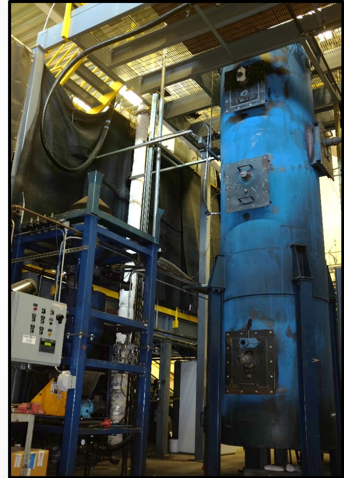
AMCD's Multi-Pollutant Control Research Facility (MPCRF)
