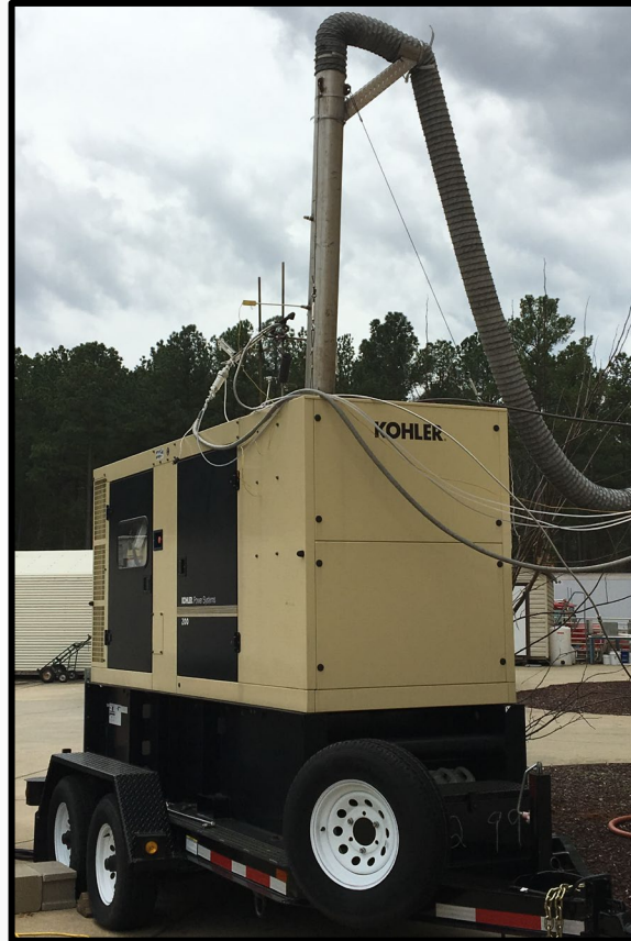
AMCD's Stationary Diesel Facility (200kW genset)
