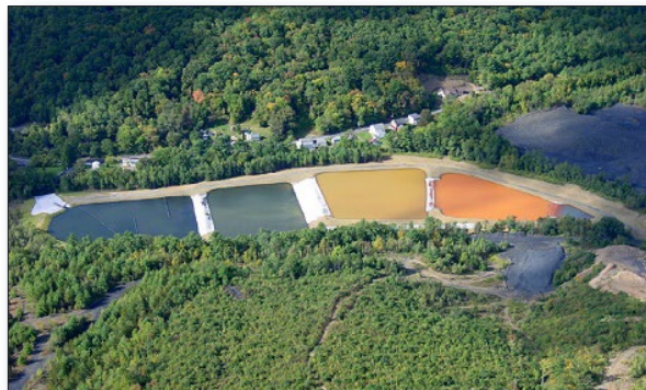
Figure 2. Partners installed an AMD passive treatment system on Silver Creek (a tributary).
