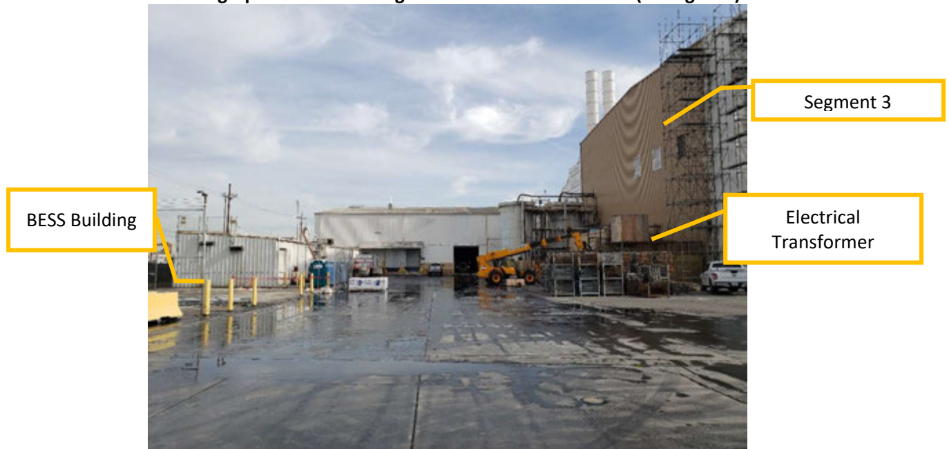
Photograph 1: BESS Building and Electrical Transformer (Facing East)
