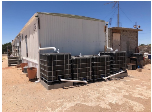
Rainwater harvest system at mobile home in Cochran Colonia, El Paso County, Texas.
