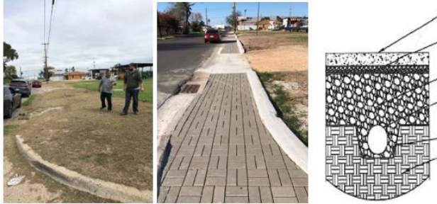
Before and after photos of high priority location, including engineer design of cross section of permeable pavement
