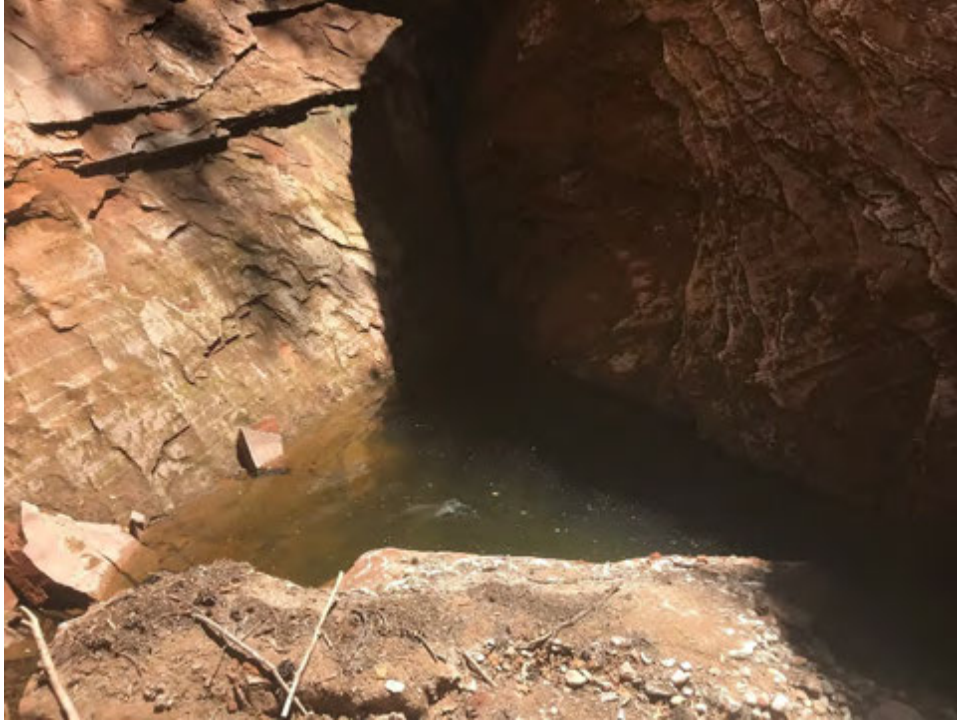
Figure J5-42. DC3A: Ponded water in drainage near SD8
