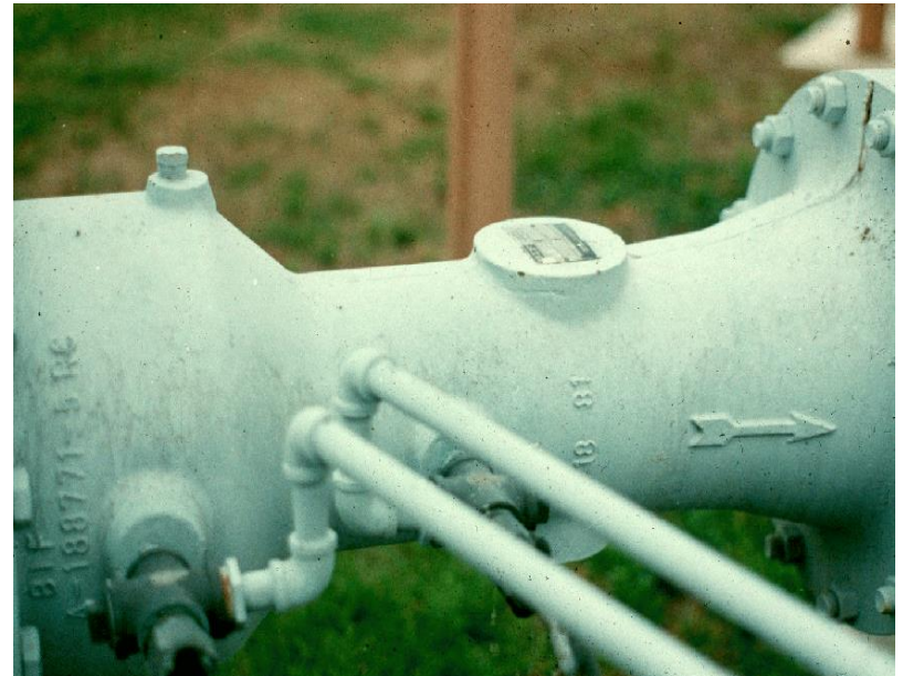
Venturi meter in operation
