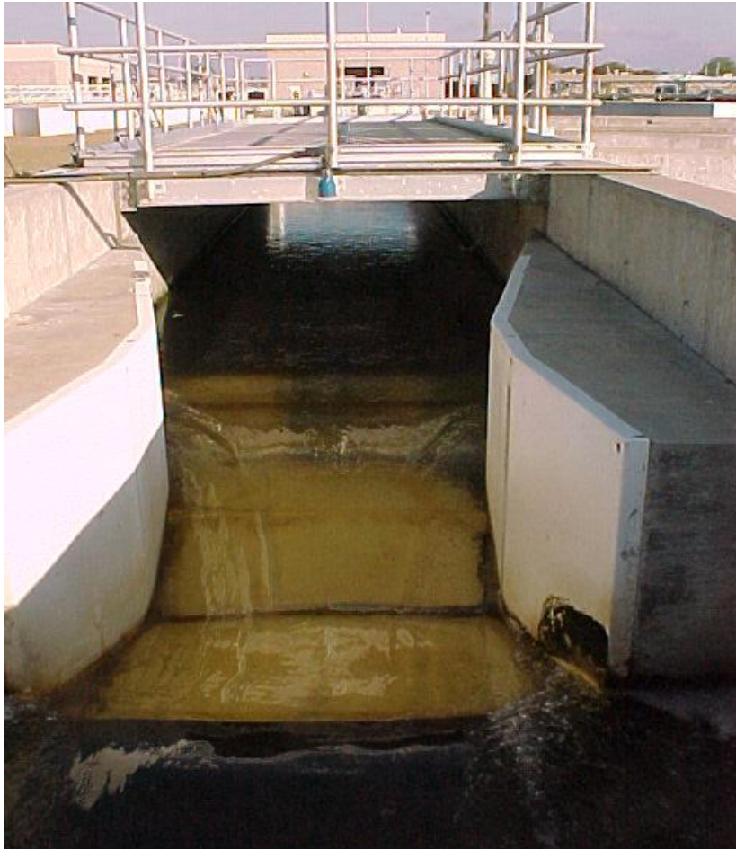
Primary Device (Parshall Flume)
