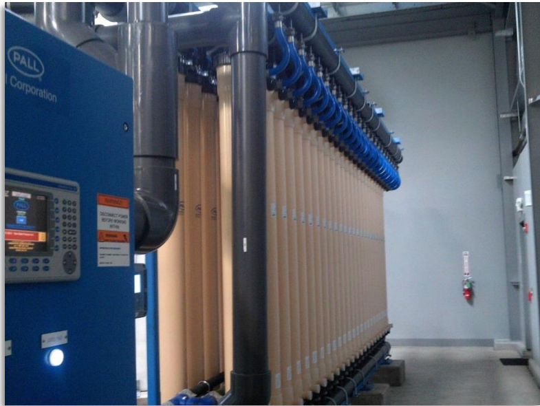
A skid of microfiltration filters
