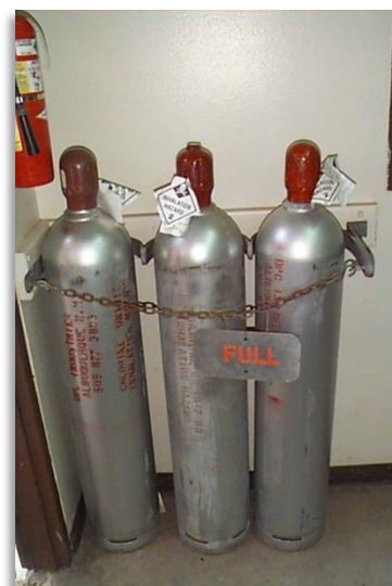
Chlorine gas cylinders
