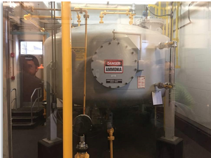
Ammonia used to form chloramines
