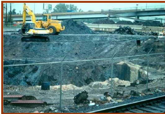
View north across one of the excavations made during Site cleanup. The North Temple viaduct is visible in the background, and the original Union Pacific railroad tracks are visible in the foreground.
