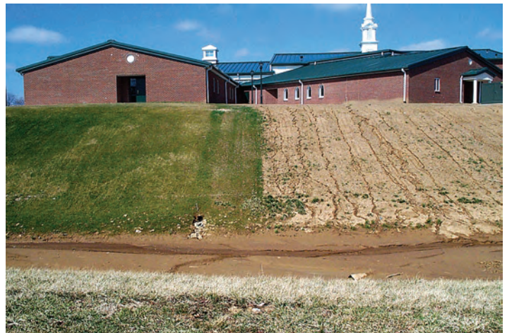
Figure 16. Seeding is an effective BMP that can be used to temporarily or permanently stabilize disturbed areas.
