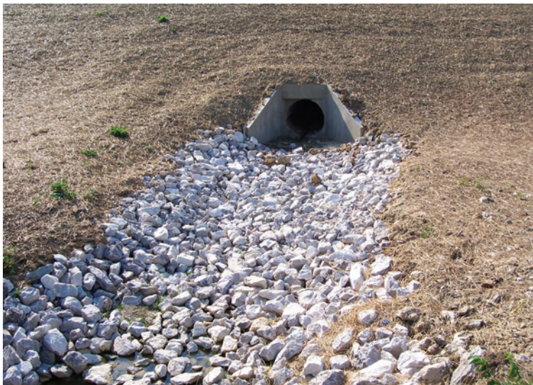
Figure 17. Make sure inlets, outlets, and slopes are well stabilized before leaving the site and filing your "Notice of Termination" for ending permit coverage.
