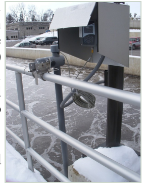
Aeration is energy-intensive process. Close monitoring of dissolved oxygen is essential.
