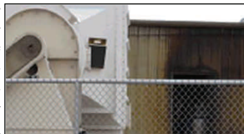
Building with heavily stained exterior as a result of the nitrogen oxide fumes.
