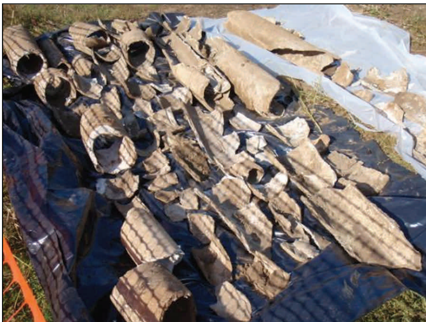
Pieces of the old cement asbestos pipe that was improperly handled by Greiner and Eberhart.
