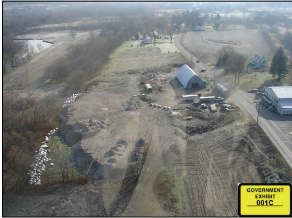
Property on the Mohawk River where thousands of tons of asbestos-contaminated construction and demolition debris was illegally dumped.
