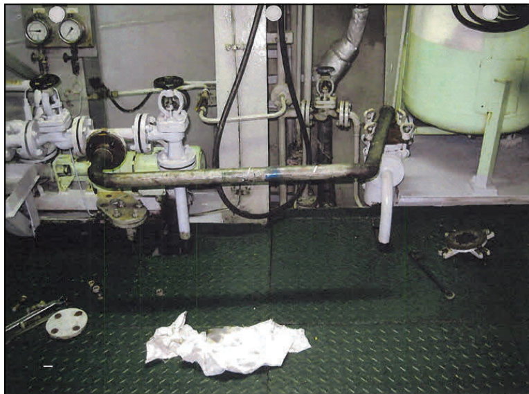
The “magic pipe” that would bypass the oily water separator and discharge oil-contaminated waste water.
