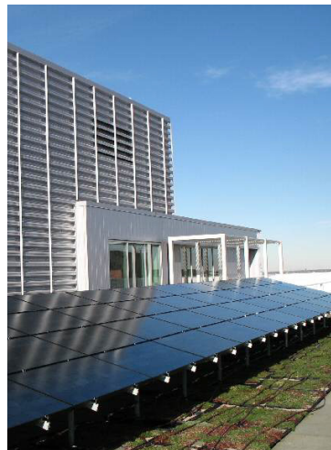
Solar panels on a green roof
