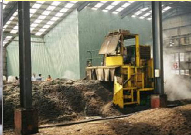
5. 堆肥場 Composting Treatment
