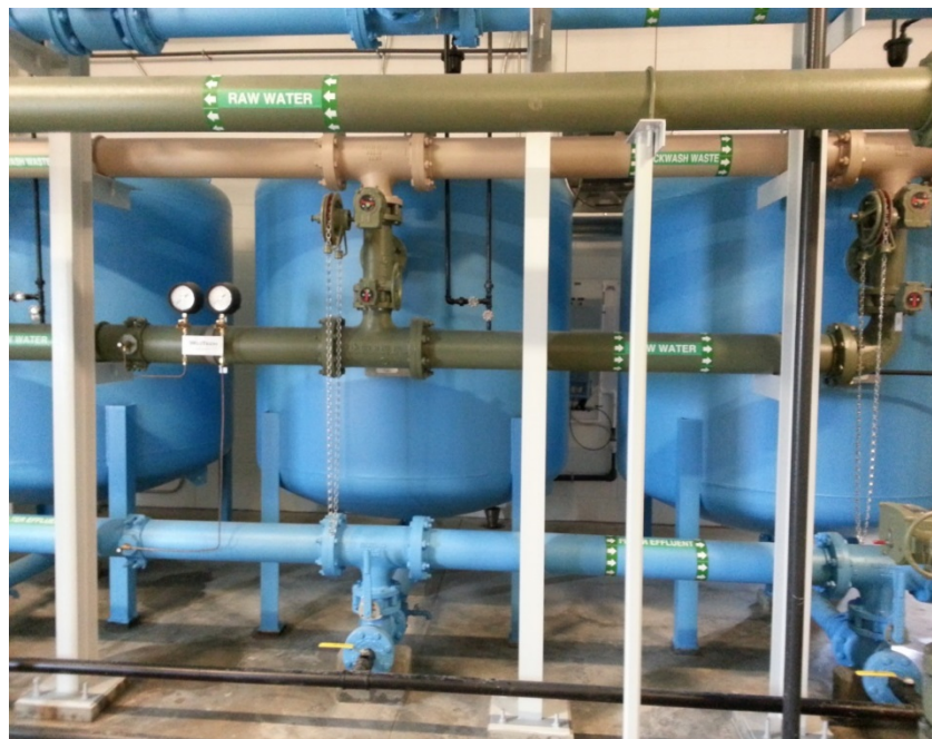
Figure 7. Photograph of pressure filters.
