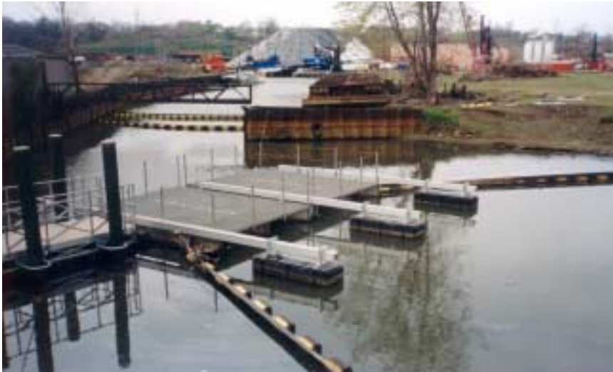
Kingsbury Run End-of-Pipe Netting Facility for control of floatables.
