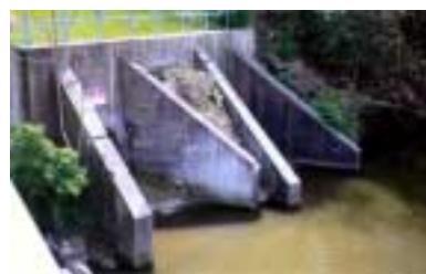
Right – Outlet structure with CSO outlet on the left, storm sewer outlet on the right.
