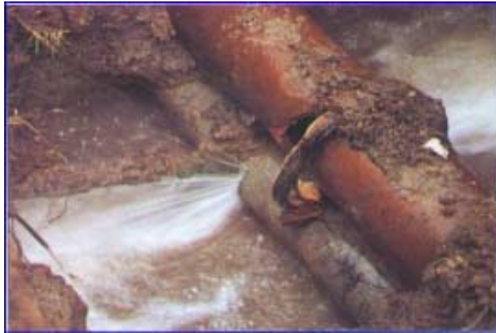
Figure 4. Leaky water pipe laid next to a sewer pipe (Source: Opflow 1999)
