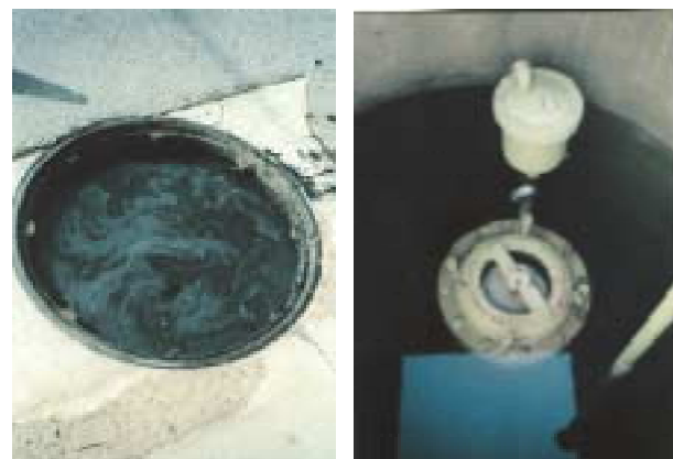
Figure 2. Submerged air release valve
