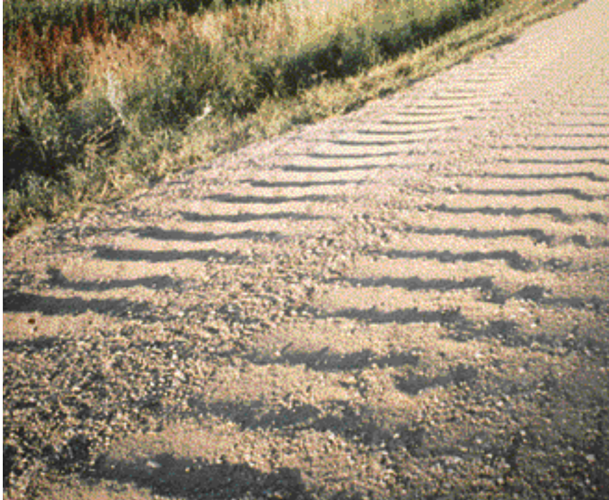
This type of corrugation, "washboarding," is caused by lack of moisture, hard acceleration, aggressive braking, and poor quality gravel.
