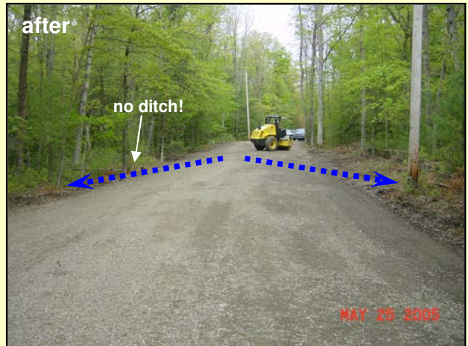
Photo 4. The road was elevated to eliminate the ditch on the left and achieve sheet flow. The added material also provided the necessary cover to install new crosspipes.
