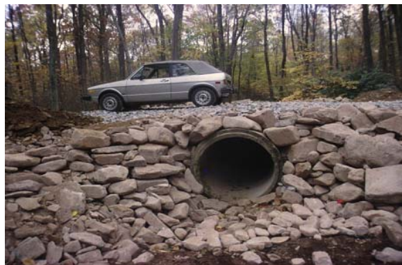
5-43 Stream Saver System – raised level road with ditch turnouts to vegetative filters.
