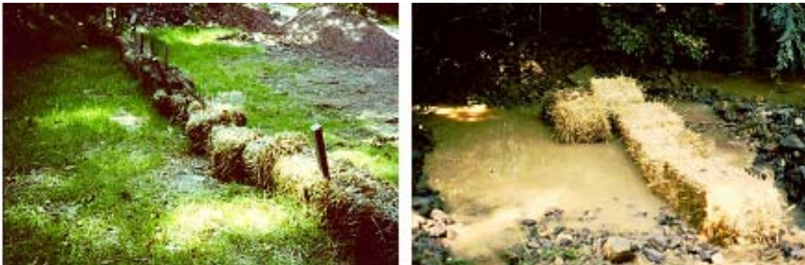
5-03 Improper bale installations doomed to fail!
