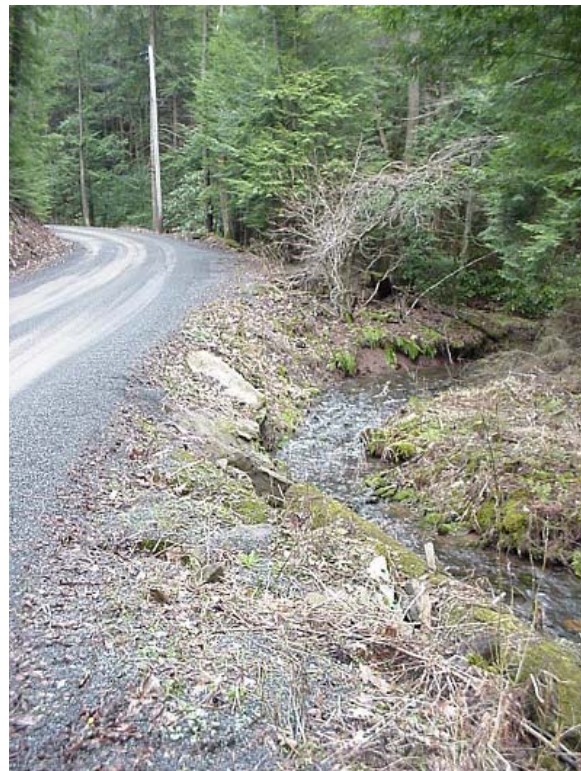
6-01 Typical roadside erosion problems.
