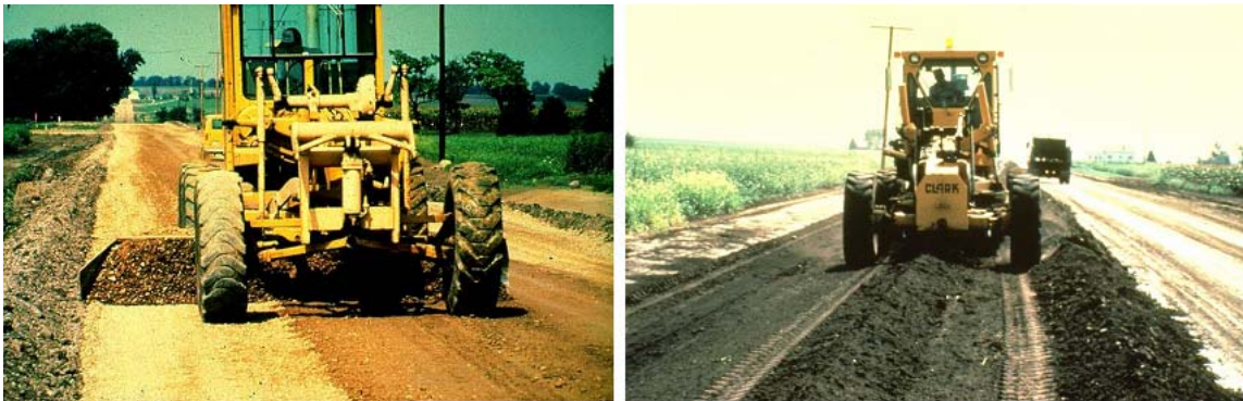
7-11 Stabilization can be accomplished with a road grader – scarifying the road, mixing in a stabilizing agent, regrading and shaping.
