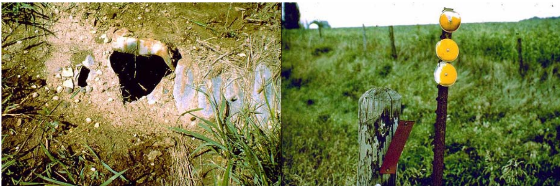
3-27 Operators should note existing problems.
