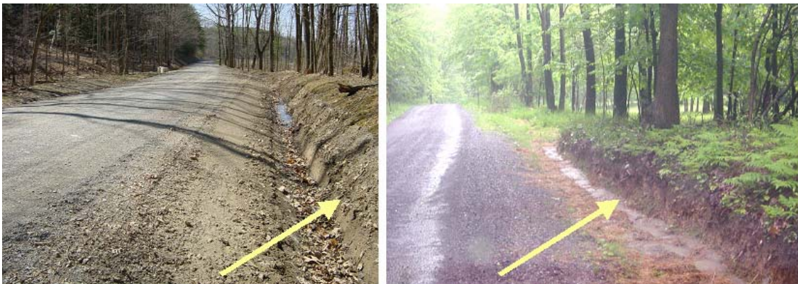
6-25 Unstable vertical bank will collapse.
