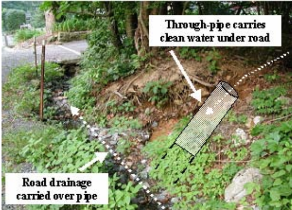
5-40 Through drains keep springs and spring seeps out of road drainage facilities.
