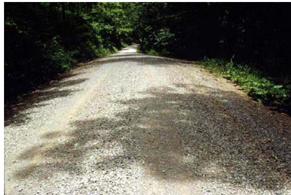
3-07A good road crown is our first line of defense against water.
