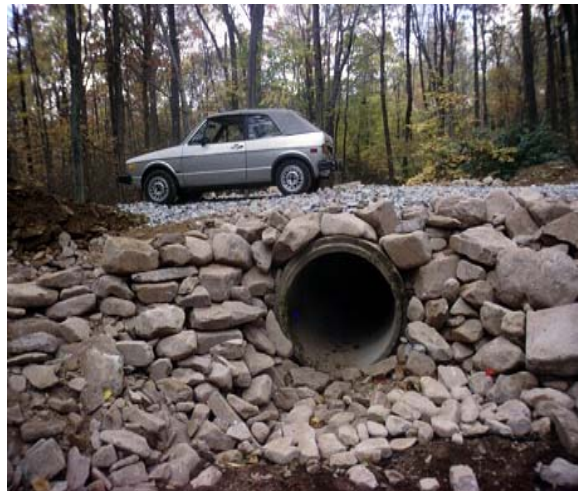
ESMP#11-01 Stream Saver System – raised level road with ditch turnouts to vegetative filters.
