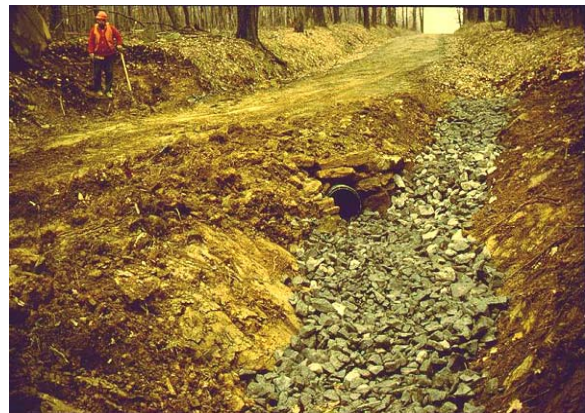
5-18 Riprap placed during construction—looking at the sediment potential, was this a good idea?
