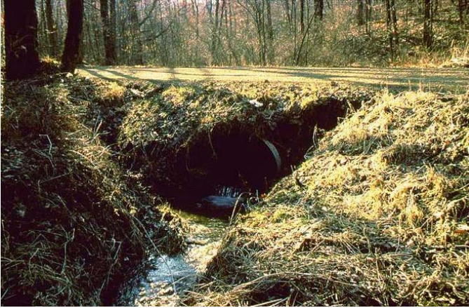
5-19 Do not outlet ditch directly to stream—use turnouts into vegetative filter strips!
