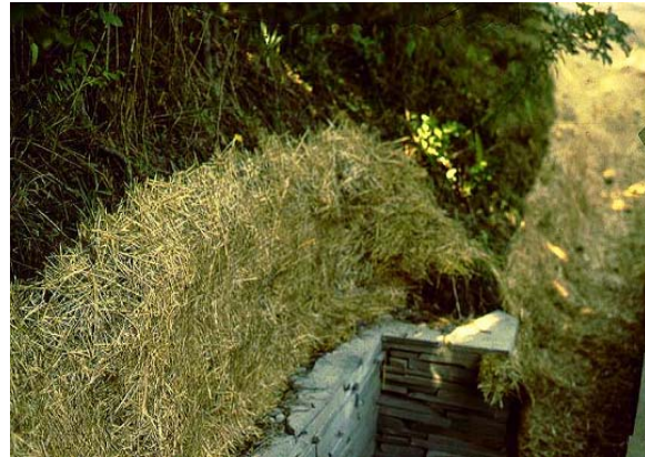
6-33 Rolled seed-impregnated straw blankets can be pinned to steep slopes for re-establishment of vegetation.
