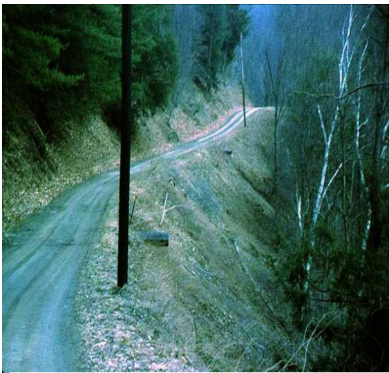
5-24 Grade breaks result in short road sections with reduced water volume and flow velocity.
