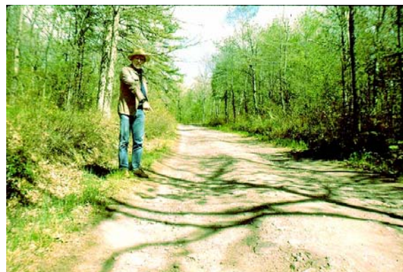
5-01 Typical entrenched eroded road.
