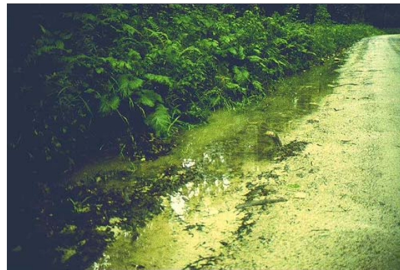
ESMP#3-01 Standing water can only lead to problems!
