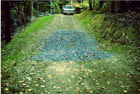
ESMP#3-02 Broad based dip reinforced with large aggregate.
