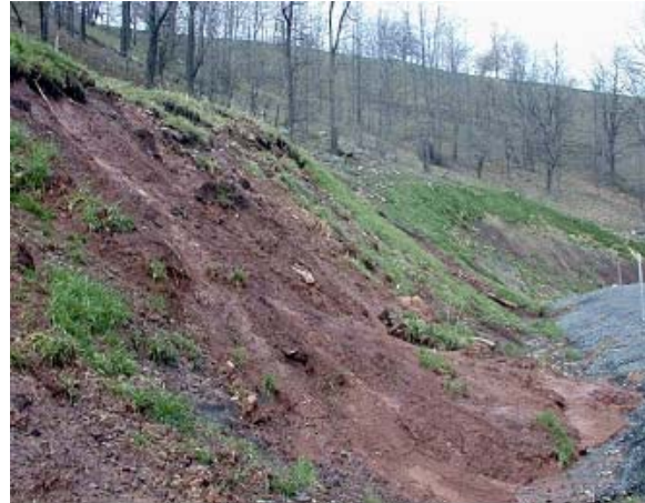
2 - 04 The relentless force of gravity causes bank failures, downed trees, loss of road gravel and water erosion.
