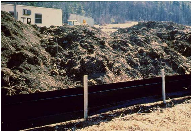
5-06 This installation will not control much sediment!
