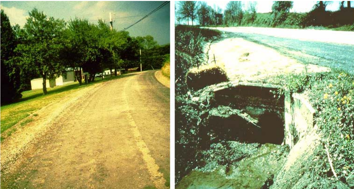
7-09 With the use of asphalt “oils,” tracking and/or run-off can become problems.
