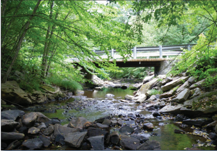
Figure 2. Restoration efforts have improved water quality in Johnson Run (looking downstream, above the confluence with East Branch Clarion River).
