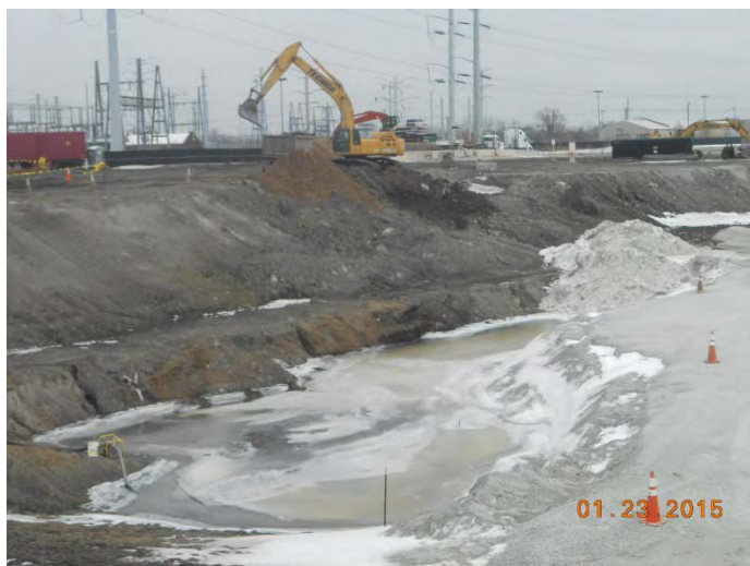
Photo 2: Tecnica pumping wastewater from the former River excavation to the on-site WWTS.
