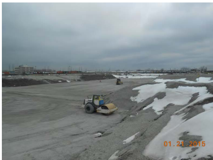
Photo 1: Tecnica continues to compact CA-6 backfill in Area 4E and the former River excavation.
