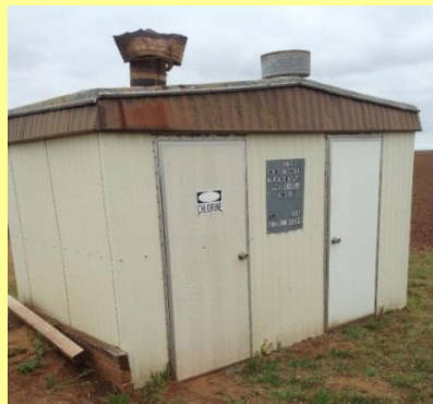
City of Weinert Water System: Wellhead (EPA OIG photo)
