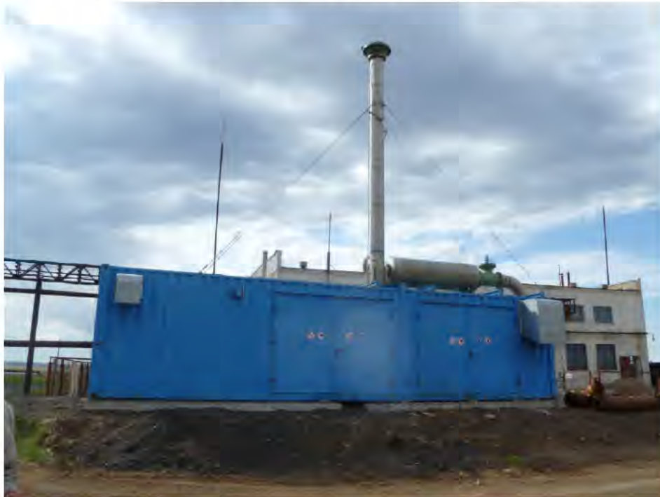
Figure 7. Positive displacement (PD) blower extraction station
