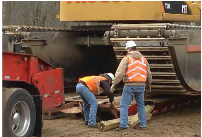
Ruben Rodriguez (left) and another employee are preparing to unload heavy equipment at the job site while responding to an oil spill on the Kalamazoo River in Michigan.
