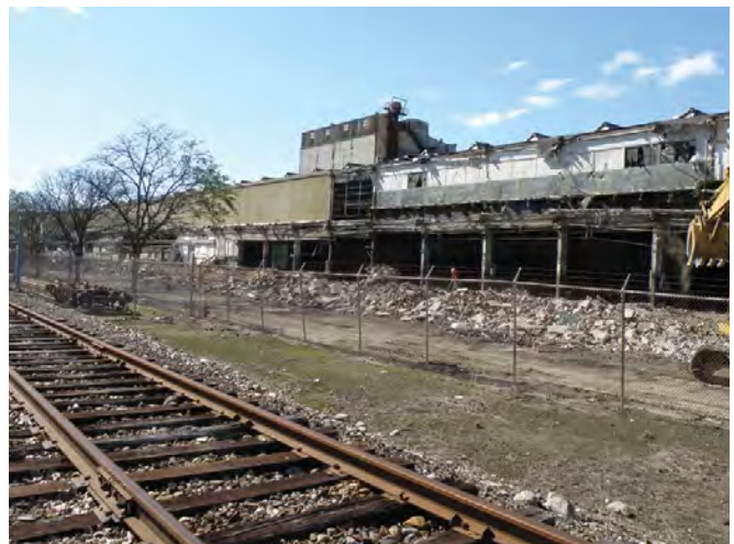
NRWIB graduates have helped salvage structural steel and concrete from abandoned buildings like this one at the Waterbury Industrial Commons.
