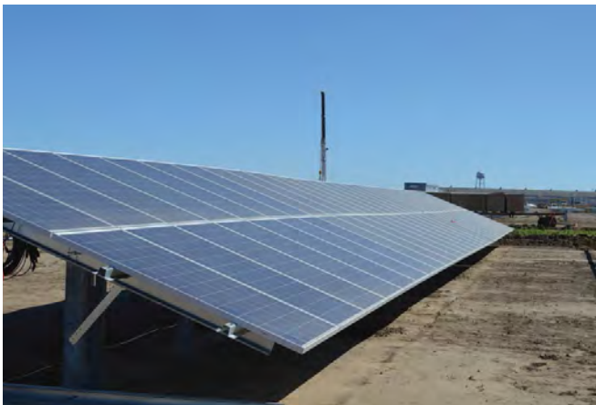
RichmondBUILD graduates helped install solar panels at the Baker Electric solar farm. The facility will use 85,000 solar panels to generate electricity that will feed directly into the Pacific Gas & Electric utility grid.
