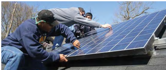
Program participants learn techniques for constructing a solar array on a roof deck rack and installing solar panels, modules and components.
