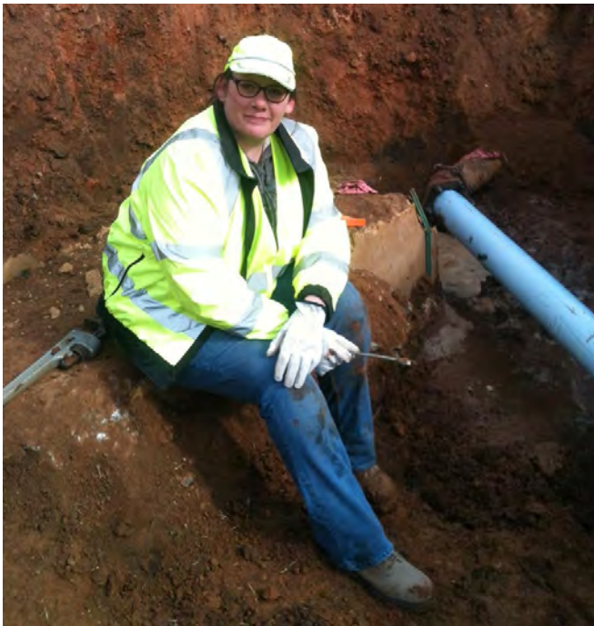
Kami Witt making water line repairs for the City of Bethany Water Treatment Plant.
