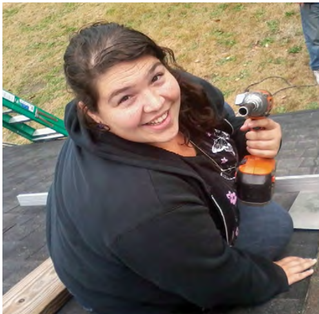
Graduate Carolyn Contravo attaching racks to a roof during her solar panel installation training. Contravo credits EPA’s environmental job training program for inspiring her interest in solar power—and for getting a job in that industry.
