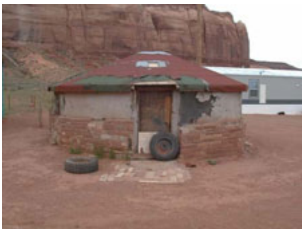
Hogan with Contaminated Foundation
