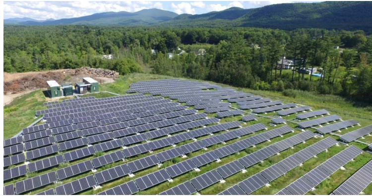
Stafford Hill Solar Farm, with the battery station visible in the left corner. Photo courtesy Green Mountain Power.
