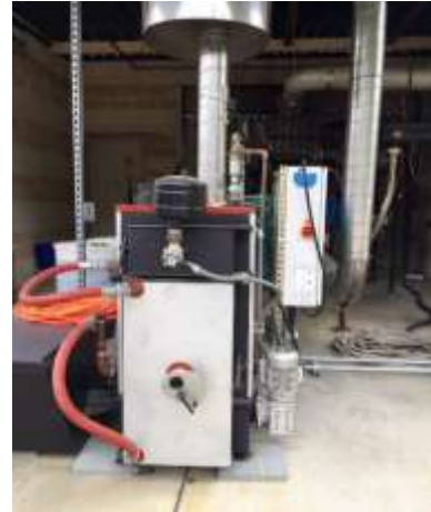
Wood-burning hydronic heater that EPA tested at its facility in Research Triangle Park, North Carolina. (EPA OIG photo)
