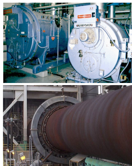
Figure 3-6. Boiler and Cement Kiln
