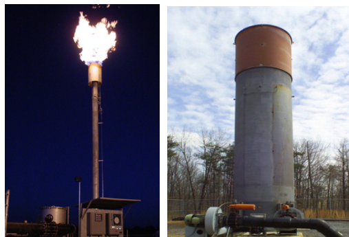
Figure 1-4. Open (left) and Enclosed (right) Flares
