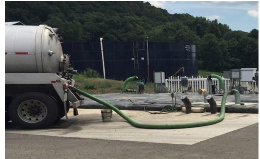
Left: Solids receiving tank with chute and steel lid
