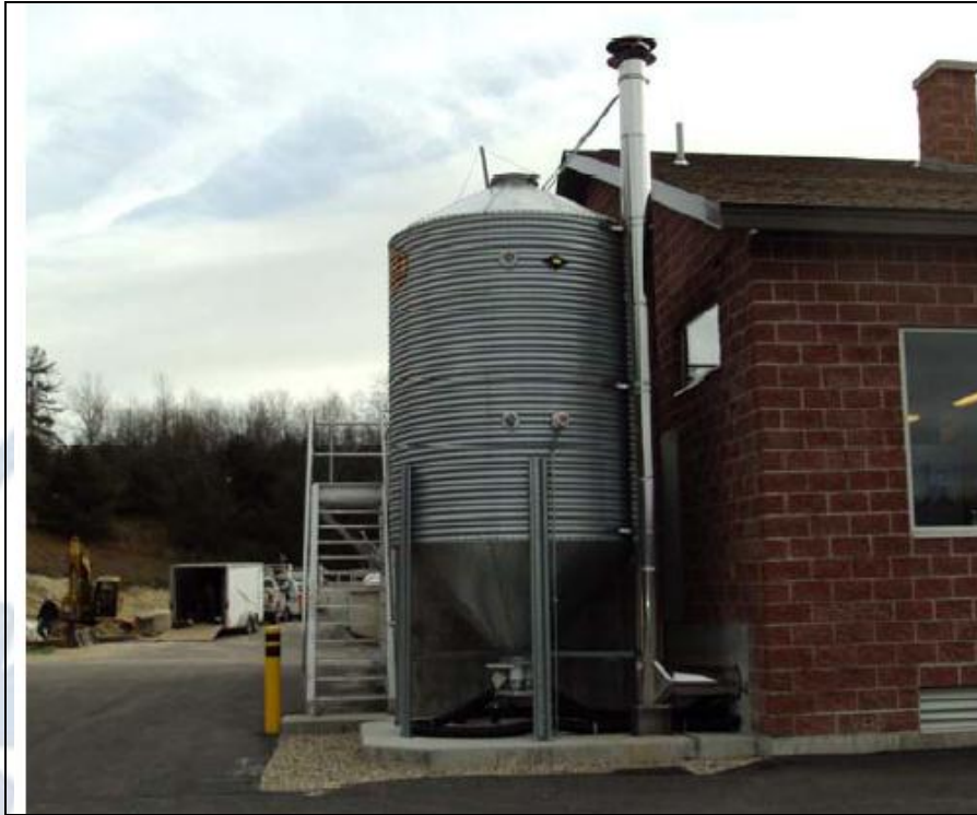
Jaffrey Wastewater Treatment Plant Pellet Silo (Source: Town of Jaffrey).
