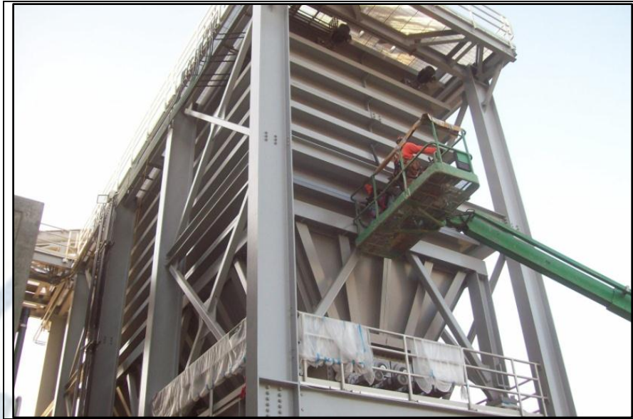
RP-1 Dewatering Facility Silo (Source: Inland Empire Utilities Authority).
