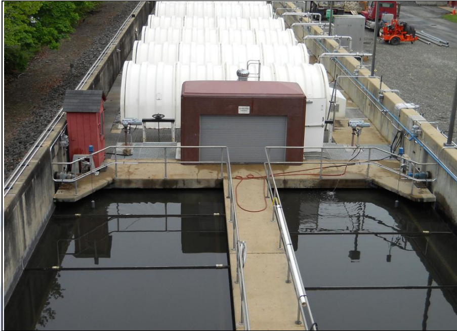
Lambertville Wastewater Treatment Plant (Source: Lambertville Sewerage Authority).
