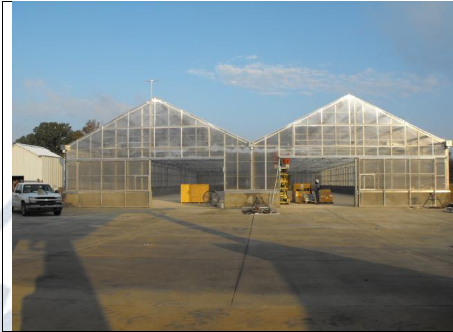
Sludge Solar Drying House Units (Source: City of Clinton).
