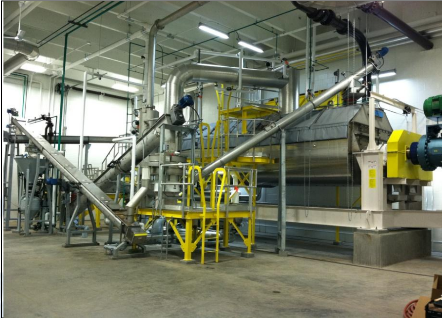
Sludge Dryer (Source: City of Big Lake).
