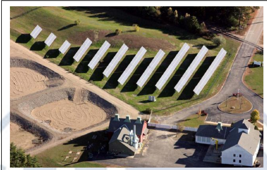
North Conway Wastewater Treatment Plant Solar System (Source: North Conway Water Precinct).
