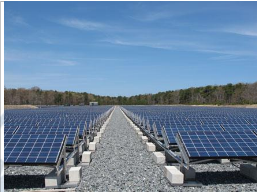
819 kilowatt Solar Array at Barnstable Wastewater Treatment Facility (Source: http://www.nexamp.com/our-projects/overview/# ).
