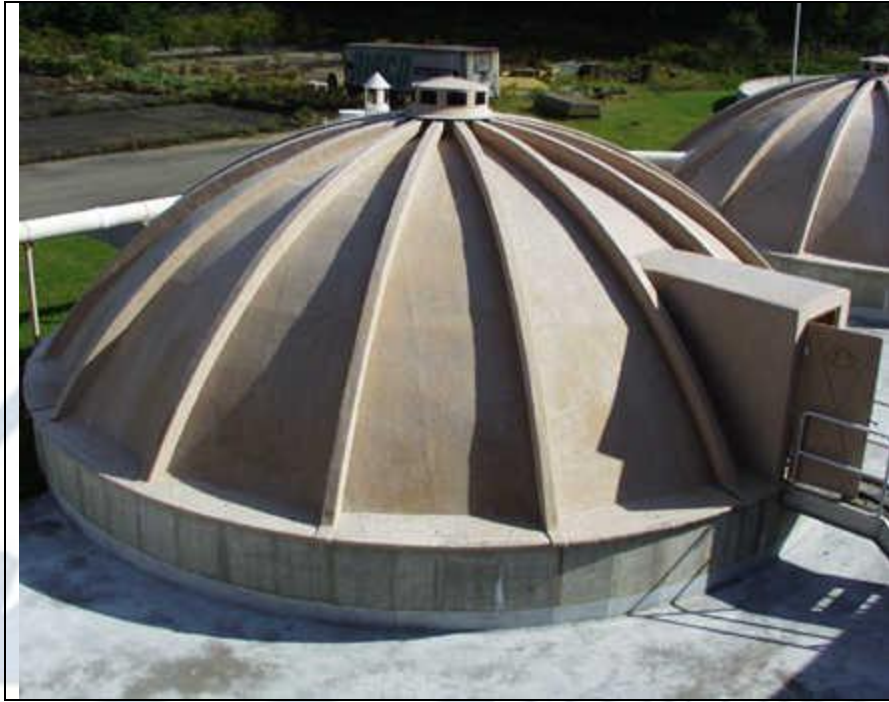
Jamestown Wastewater Treatment Plant Anaerobic Digester (Source: http://www.jamestownbpu.com/ww/tour/tour15.jpg ).
