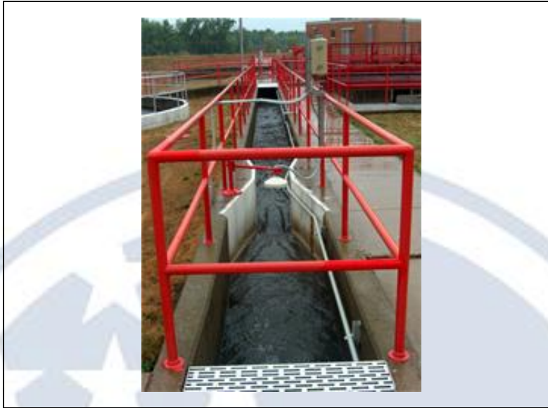
LaSalle Wastewater Treatment Plant (Source: http://www.lasalle-il.gov/content/public-works-119201081813am.aspx ).
