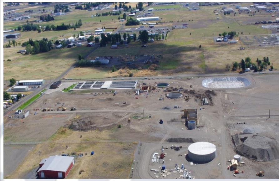
Construction of the New Wastewater Treatment Plant (Source: Century West Engineering Corporation).
