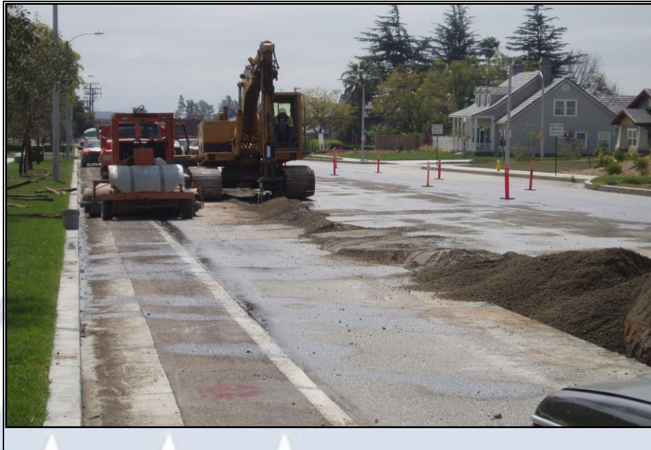
Backfill of Church Street Lateral Pipeline Trench (Source: Inland Empire Utilities Agency).
