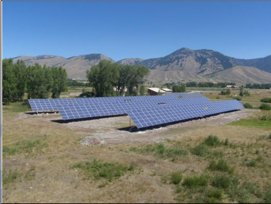
165 kW solar panel array (Source: Town of Jackson – Public Works).
