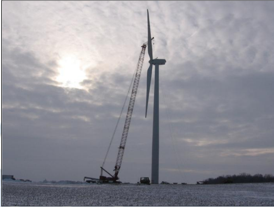
Wind Turbine (Source: City of Osage).
