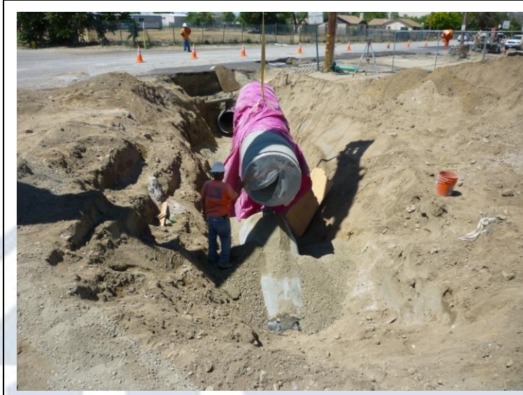
36-inch Recycled Water Pipeline (Source: Inland Empire Utilities Agency).
