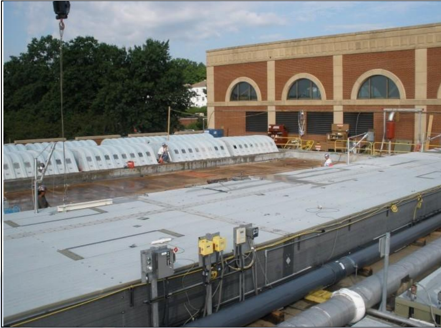
Mamaroneck Wastewater Treatment Plant Aeration Tank (Source: http://www.carlincontracting.com/projects/detail/17/Wastewater-Treatment-Plant-Nitrogen-Removal-Improvements-Mamaroneck-NY )
