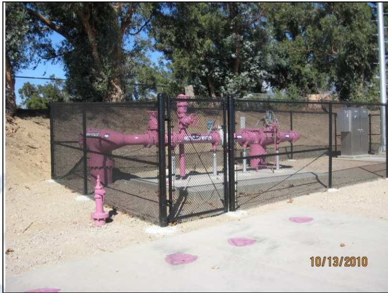
Pipeline turnout at San Sevaine Basin (Source: Inland Empire Utilities Agency).
