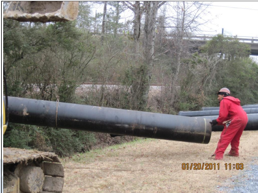
Replacement of Existing Collection System Assets (Source: Childersburg Water Works, Sewer & Gas Board).
