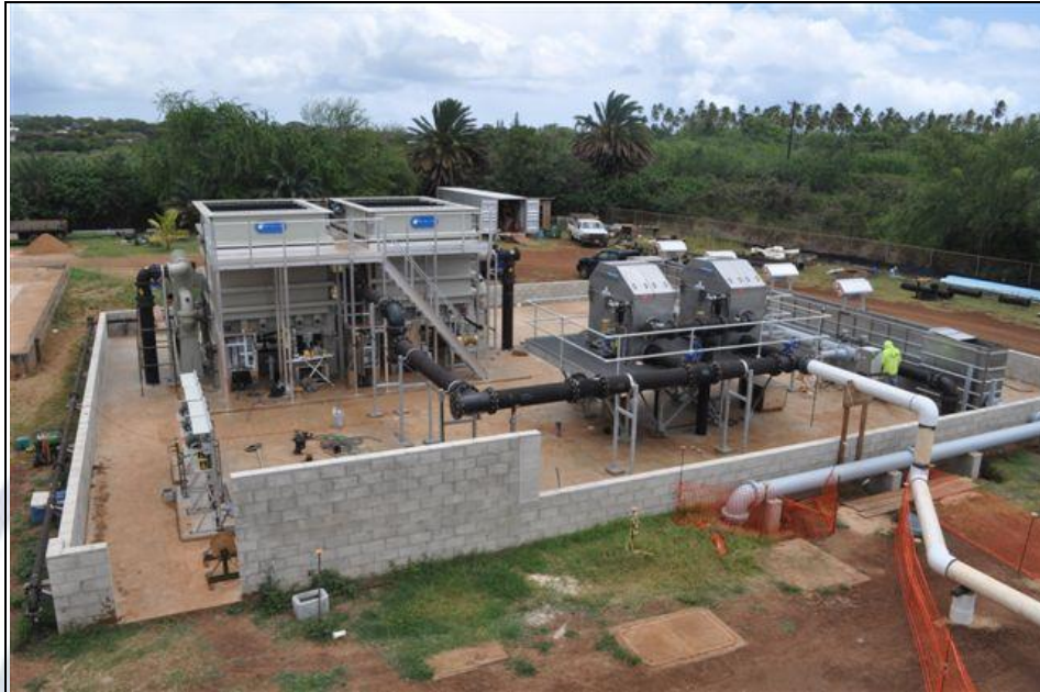
Waimea Wastewater Treatment Plant Tertiary Treatment Units (Source: County of Kauai).
