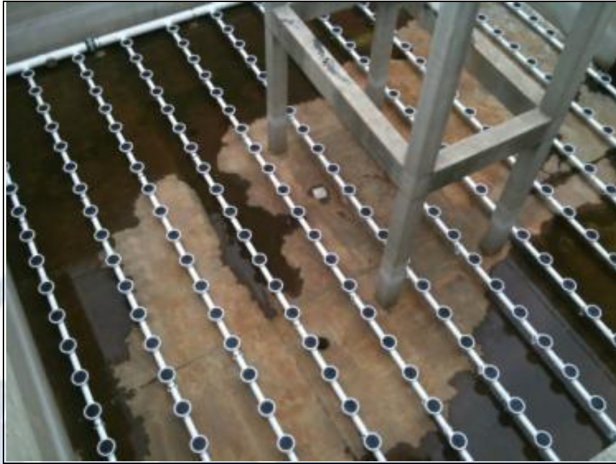
Fine Bubble Aeration Diffusers (Source: http://www.foxeng.com/news/aeration-replacement ).
