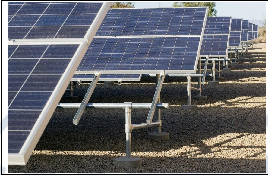
Beardsley Water Reclamation Facility Solar Array (Source: City of Peoria).
