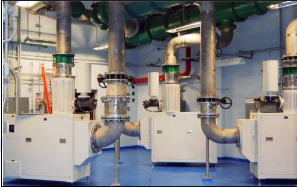
Aeration system blowers (Source: Winnepesaukee River Basin Program).
