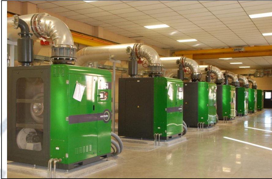
High-efficiency, turbo blowers (Source: Decatur Utilities Authority).
