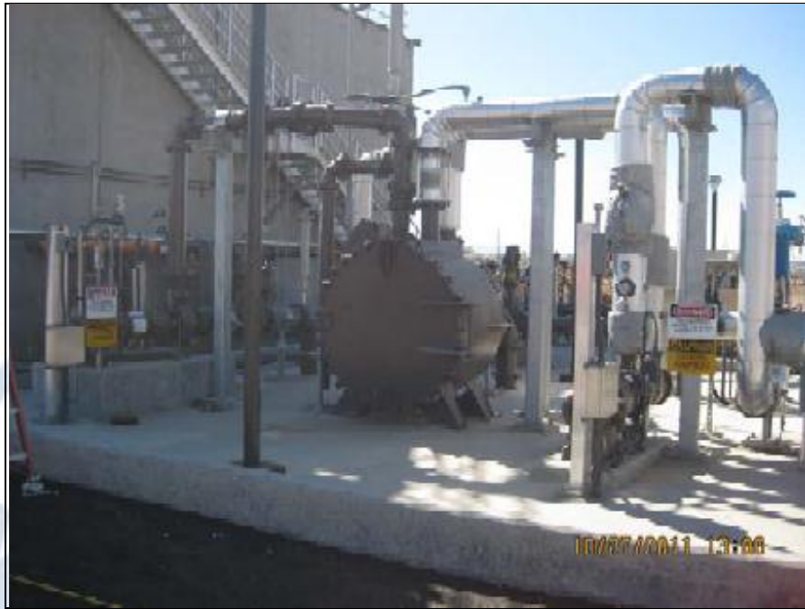
Acid Phase Digester (Source: Eastern Municipal Wastewater District).
