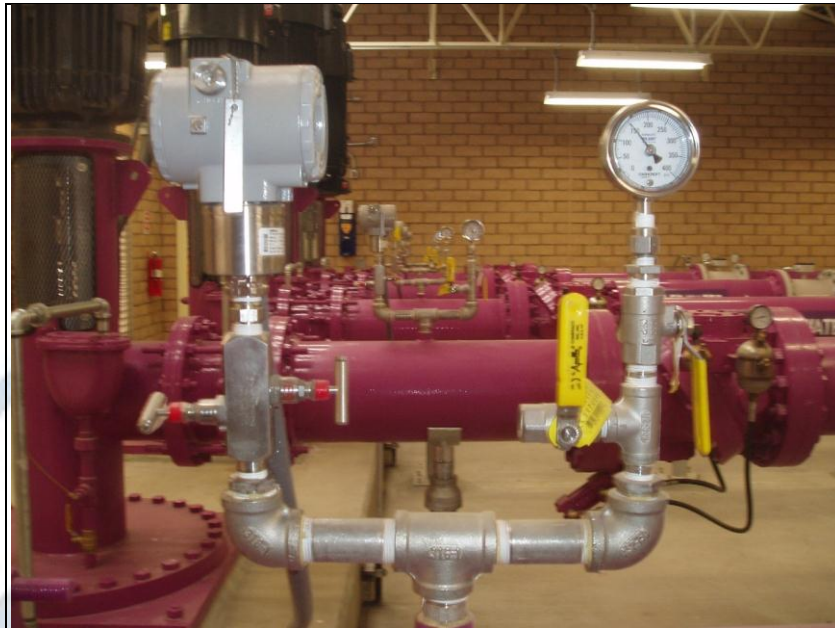
Pump Station (Source: Inland Empire Utility Authority).
