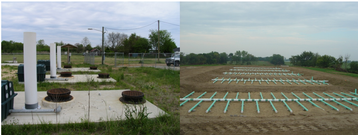
Community FAST® Units with drainfield In Virginia, USA
