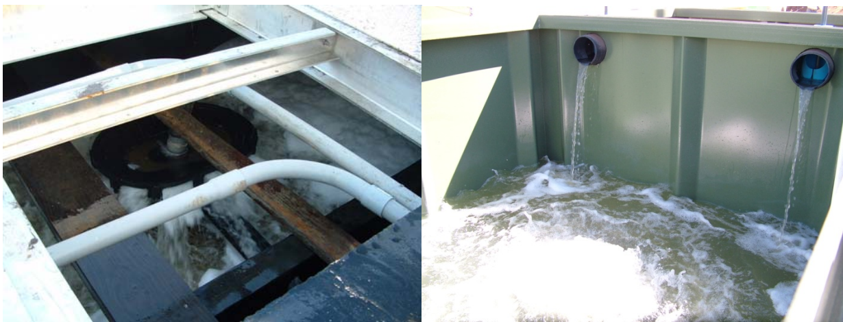
Commerical FAST® Unit in steel tank in Mexico
