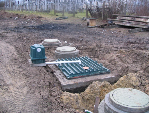
Residential FAST® System in Latvia
