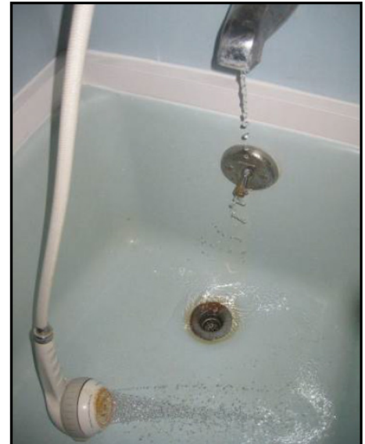
Taitem Engineering, PC, 2011. “Leaking Shower Diverters”
