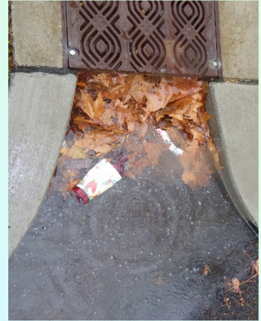
Inflow backing up due to debris and clogging
