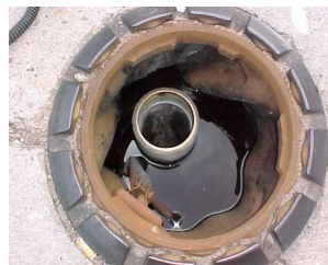
Damaged spill bucket
