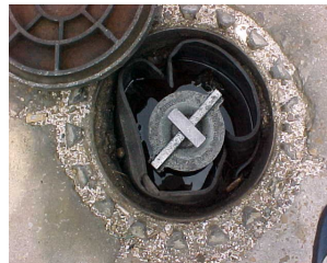
Deformed spill bucket wall
