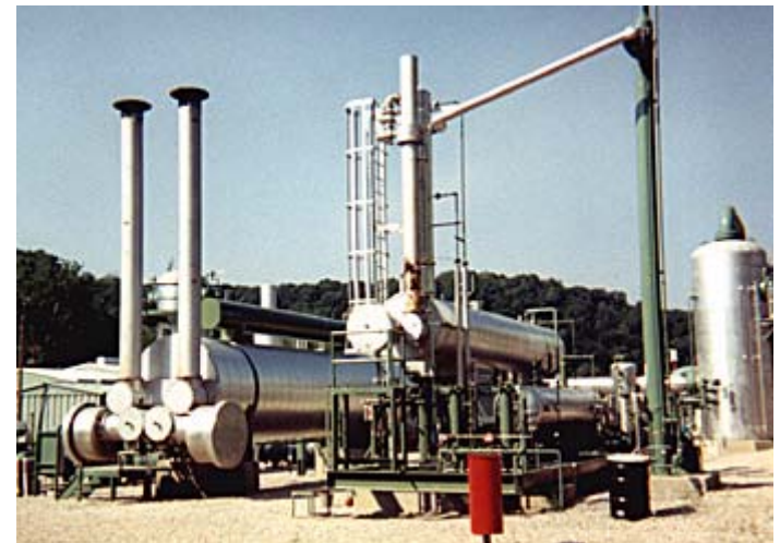
Glycol Dehydrator Unit Source: GasTech
