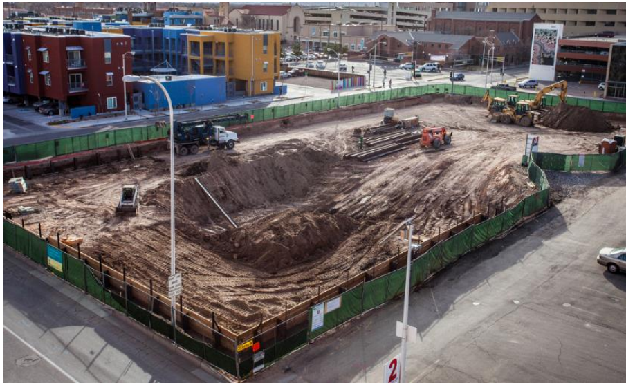
This construction site—a former brownfield site in Albuquerque, New Mexico—later became a 12,000-square-foot grocery store. (EPA photo)
