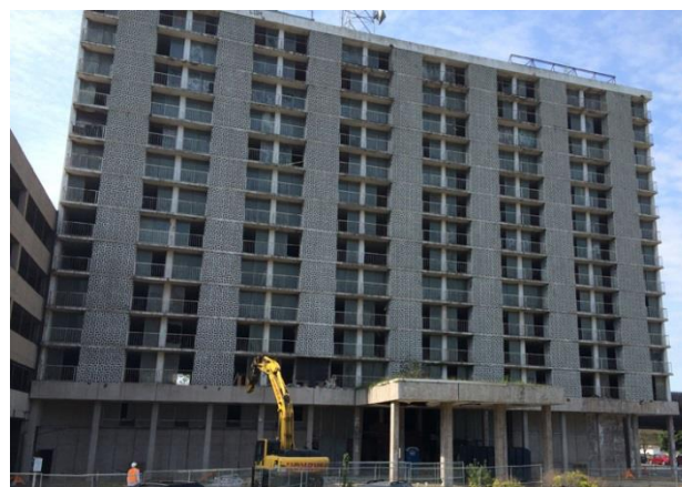
EPA Brownfields grants funded asbestos removal from an abandoned building, clearing the way for its demolition in Gary, Indiana. (EPA photo)
