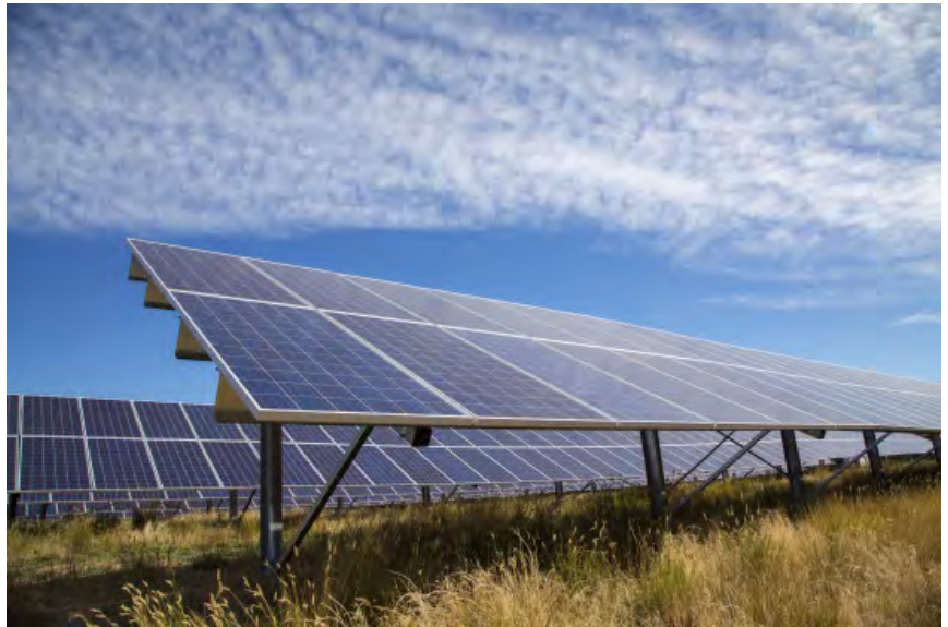
Completed Riverside Community Solar Project at the former defunct Dreher Pickle Plant site. Photo credit City of Fort Collins.
