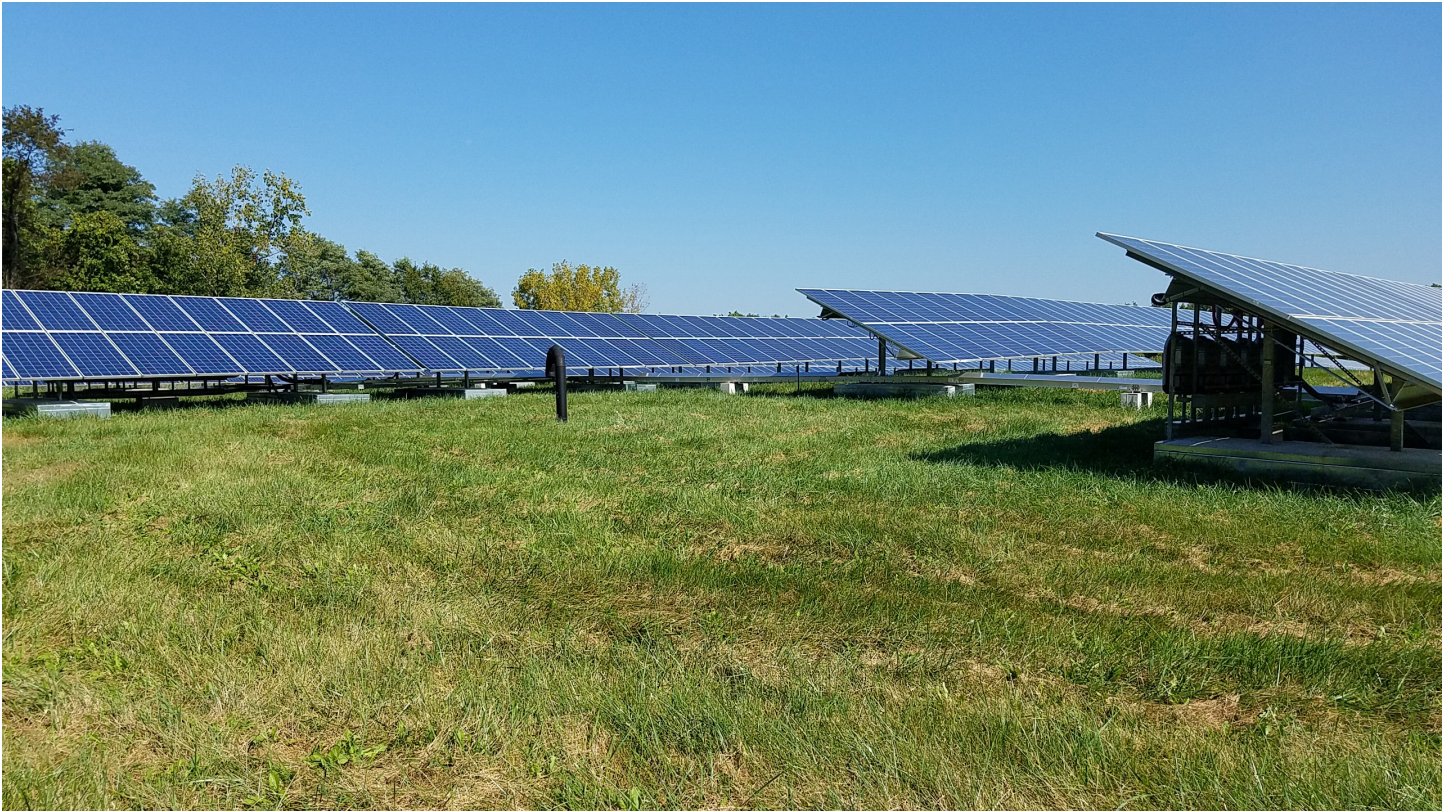
Clifton Park landfill solar installation. Photo courtesy of EPA Region 2.
