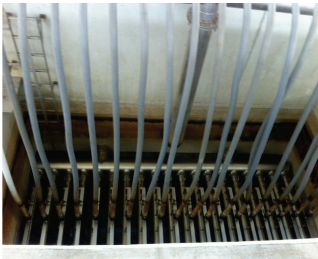
Figure 6-2. Submerged MF membranes at OCGWR
