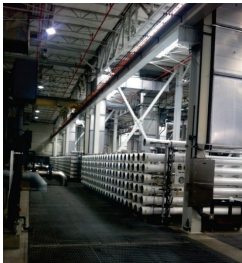
Figure 6-3. RO system at OCGWR
