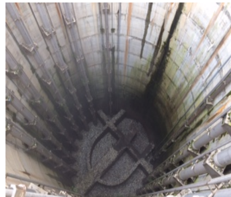
Atlanta Department of Watershed Management's West-Area Tunnel Shaft (EPA OIG photo)
