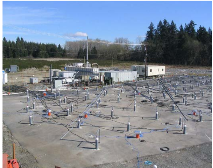
In situ thermal treatment of DNAPL using electrical resistive heating (ERH) at Fort Lewis Logistics Center NPL Site (Thermal Remediation Services, 2008)
