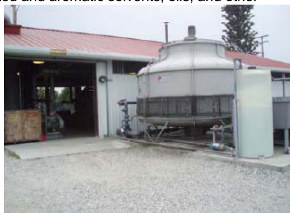
Groundwater Treatment Facility at Pemaco Superfund Site (EPA, 2010)
